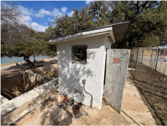
Photo #33 View of pool chemical storage shed installed at deck level.
