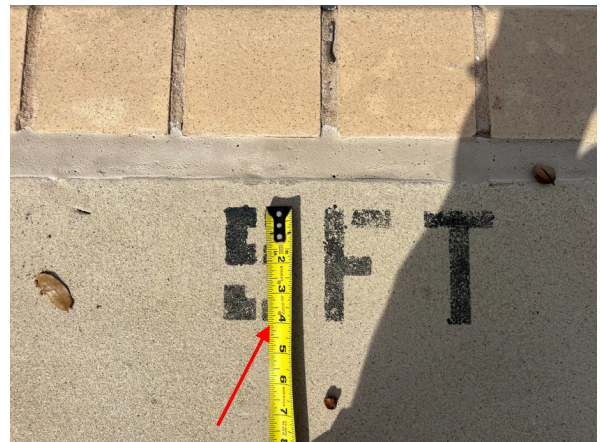
Photo #4 Example view of a 4" tall depth marking on the Lap Pool deck.
