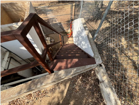
Photo #37 View of corroded stairs leading down to the main mechanical space.
