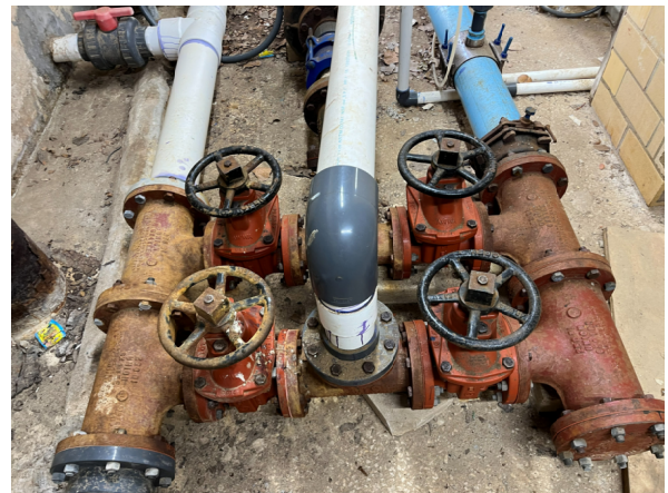
Photo #54 View Lap Pool backwash valving.
