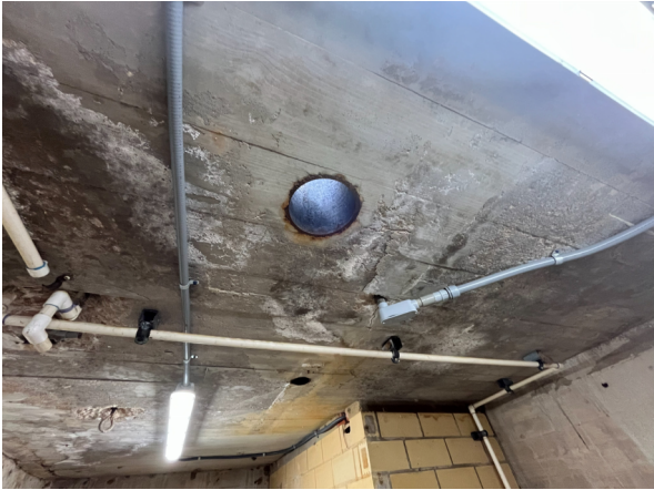
Photo #48 View ventilation/open pipe in the roof of the main mechanical space.
