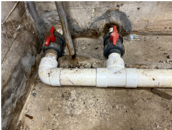
Photo #51 View of suction lines (four (4) instances) coming from the vacuum sand filter pits.
