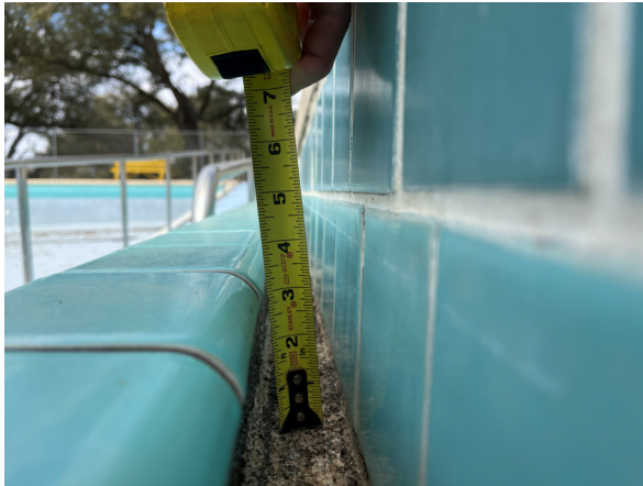
Photo #19 View of the gutter trough that runs around the perimeter of the Lap Pool.
