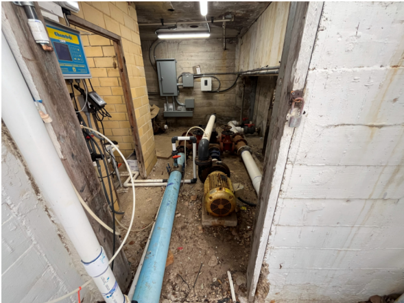
Photo #38 View of Lap Pool mechanical room.
