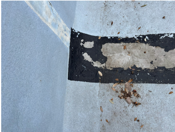
Photo #25 View of waterproofing material installed to prevent water loss in the Lap Pool. Likely covering an old construction joint in the pool floor.
