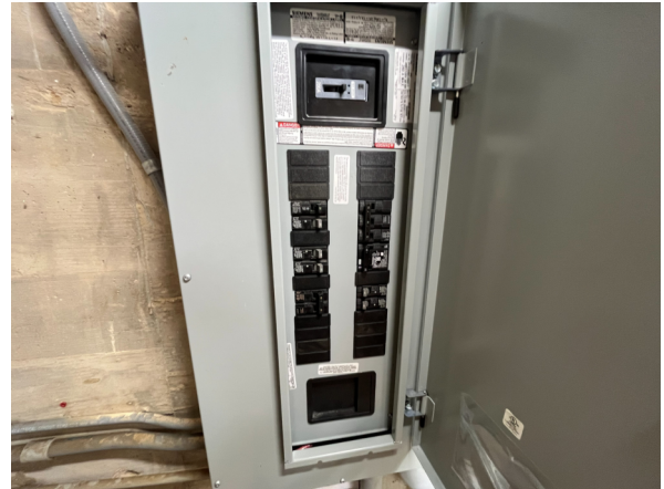
Photo #50 View of breaker panel.
