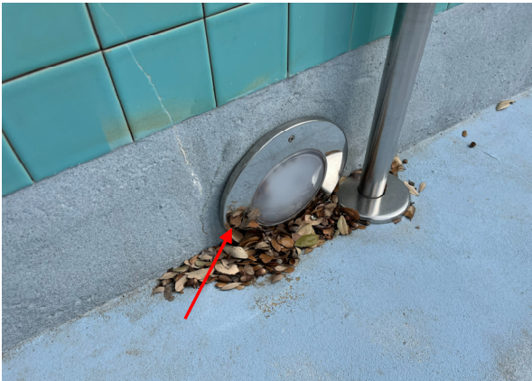
Photo #18 View of an underwater light installed in the Lap Pool ramp entry.
