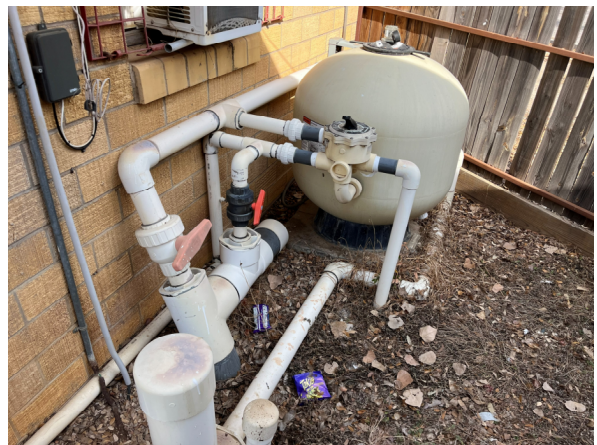
Photo #58 Example Small Pool mechanical systems.
