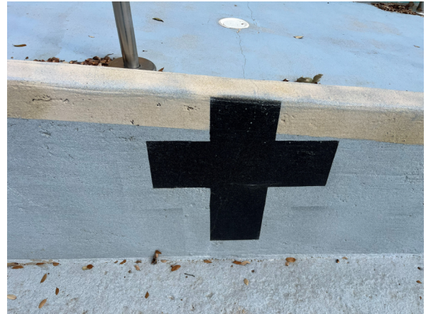
Photo #20 View of Lap Pool wall target installed beneath the ramp entry.
