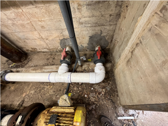
Photo #43 Example view of suction lines (four (4) instances) coming from the vacuum sand filter pits.
