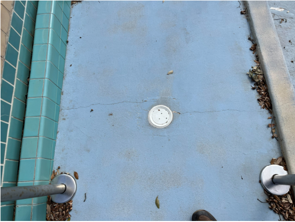
Photo #17 Example view of Lap Pool floor inlet serving the ramp entry.
