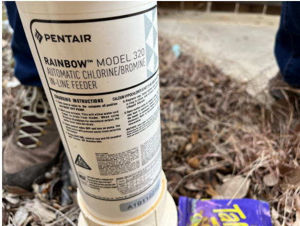
Photo #61 View of small pool inline chlorination system.
