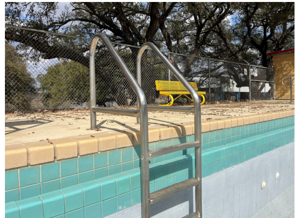
Photo #28 Example view of the grab rails installed around the Lap Pool.
