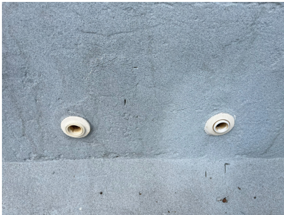
Photo #21 Example view of Lap Pool wall inlets – installed in sets of two (2).
