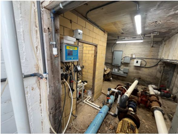
Photo #39 View of Lap Pool water chemistry controller and chlorine feed room.
