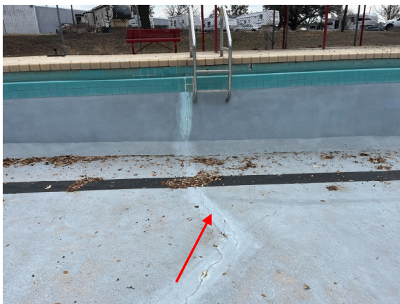
Photo #23 View of large crack that runs across the Lap Pool floor and south wall.
