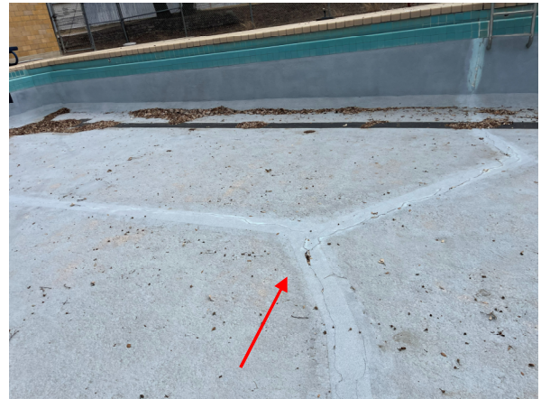
Photo #22 View of large cracks sprawled out on the Lap Pool floor.
