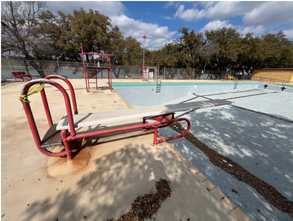
Photo #31 View of the broken diving board installed on the west side of the Lap Pool.
