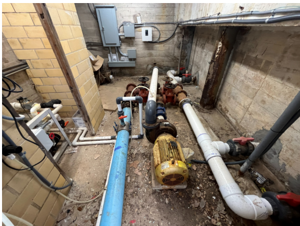
Photo #53 View of Lap Pool mechanical space.
