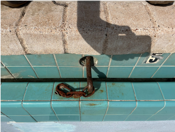
Photo #14 View of a Lap Pool wall anchor and rusted chain that appears to no longer be in use.
