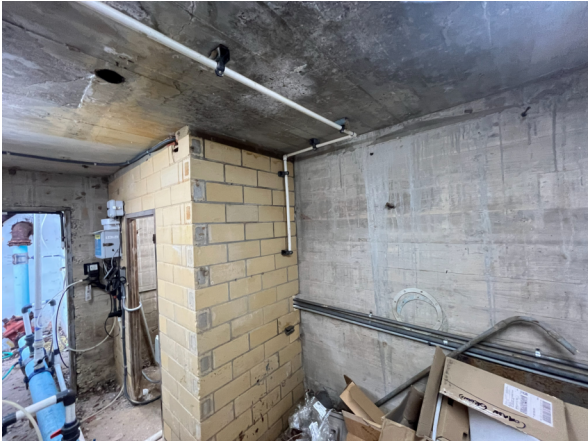
Photo #47 View of abandoned piping outside the chemical treatment room.
