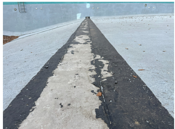
Photo #24 View of waterproofing material installed to prevent water loss in the Lap Pool. Likely covering an old construction joint in the pool floor.
