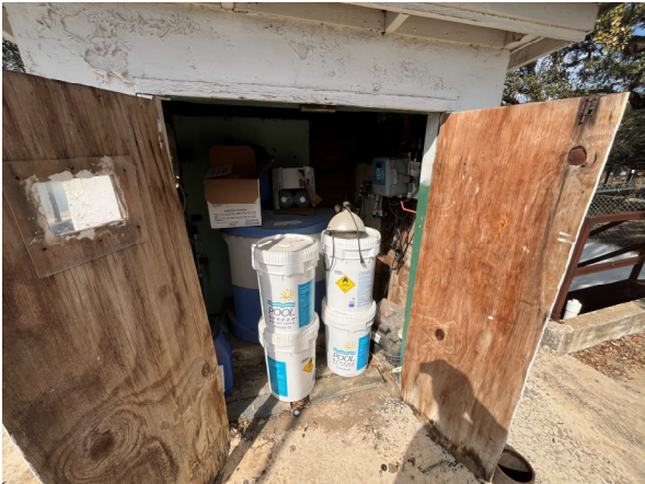
Photo #32 View of pool chemical storage shed installed at deck level.
